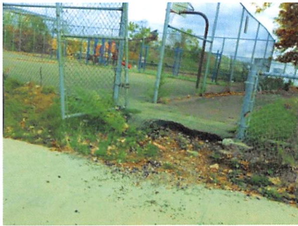
57 th Street Playground - Damaged and Inaccessible Entry Way – Rated Poor
