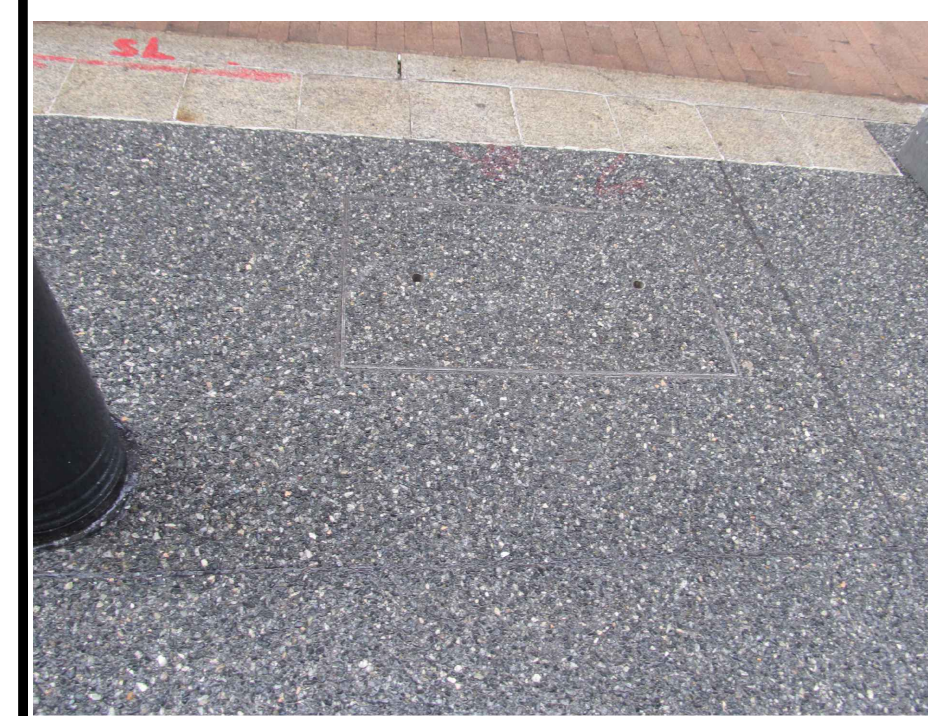
10 TRAFFIC SIGNAL ACCESS PANEL
