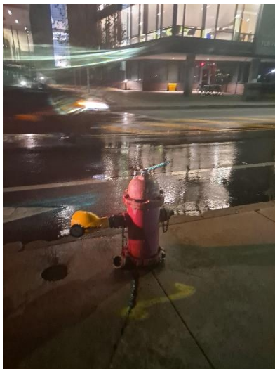
Hydrant C188 (North facing)
