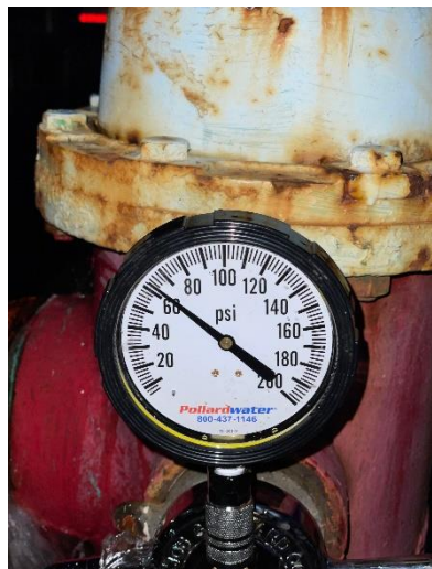
Pressure reading for hydrant C1455
