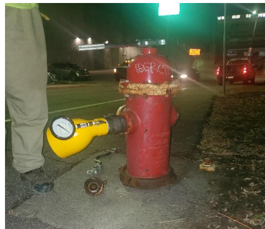
Hydrant C192 (East facing)
