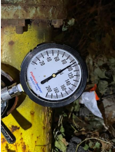
Pressure reading for hydrant C191
