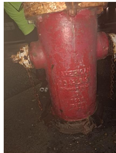
Hydrant C192 (East Facing)
