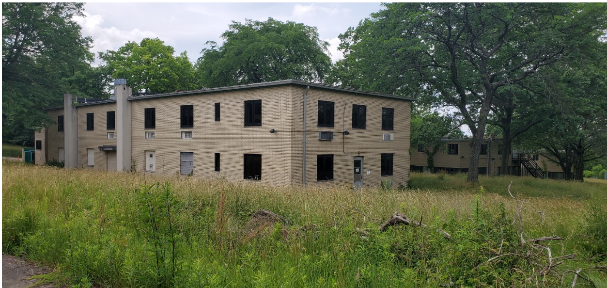
North section two-story eastern elevation with engaged concrete columns, and northern elevation
