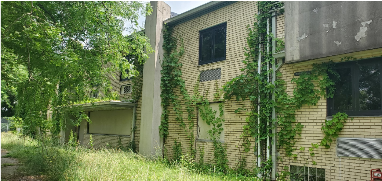
Western elevation, two-story north section with engaged concrete columns, and one-story middle bridge section with screen for HVAC
