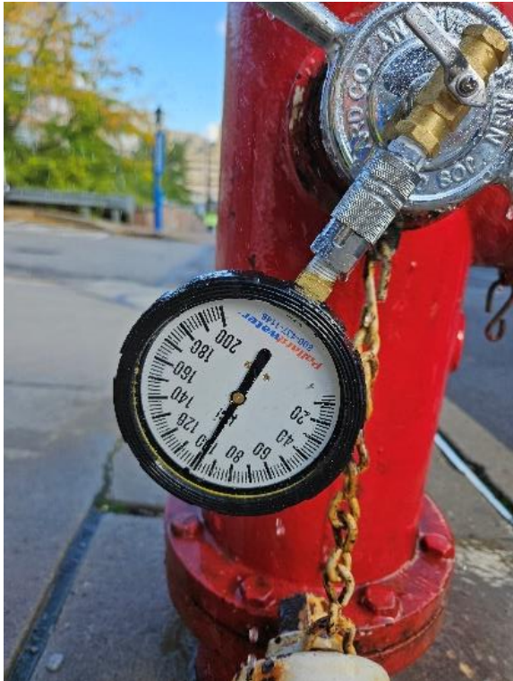
Static Pressure Reading for Pressure Hydrant
