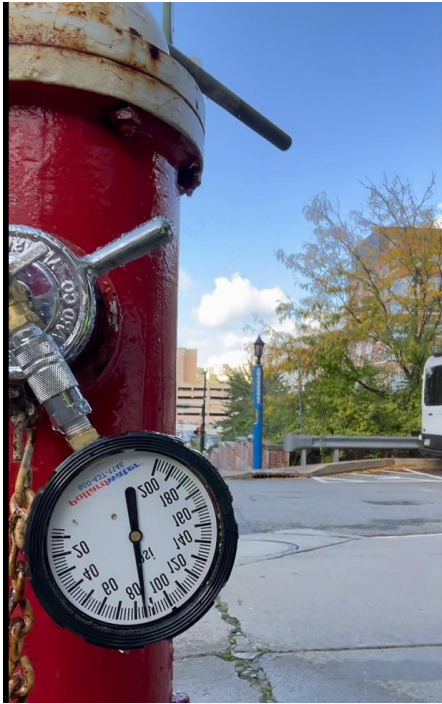
Residual Pressure Reading for Pressure Hydrant
