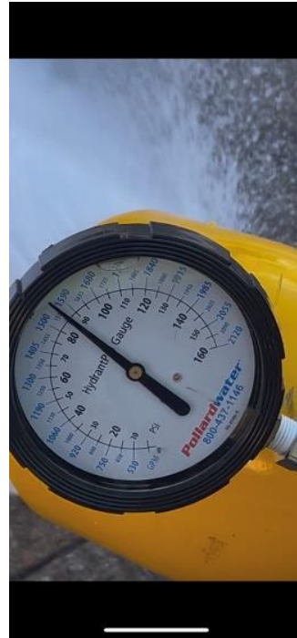
Pressure and flow reading for Flow Hydrant 1
