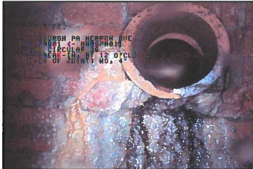
Photo: 3_6A, 00:04:49 55.5FT, Tap Break-In, at 12 o'clock, -, within 8 inches of joint: NO, 4"
