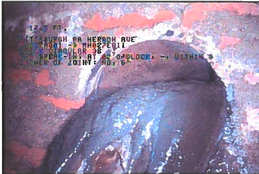
Photo: 1_4A, 00:05:42 17.5FT, Tap Break-In, at 02 o'clock, -, within 8 inches of joint: NO, 6" / DEPOSITES
