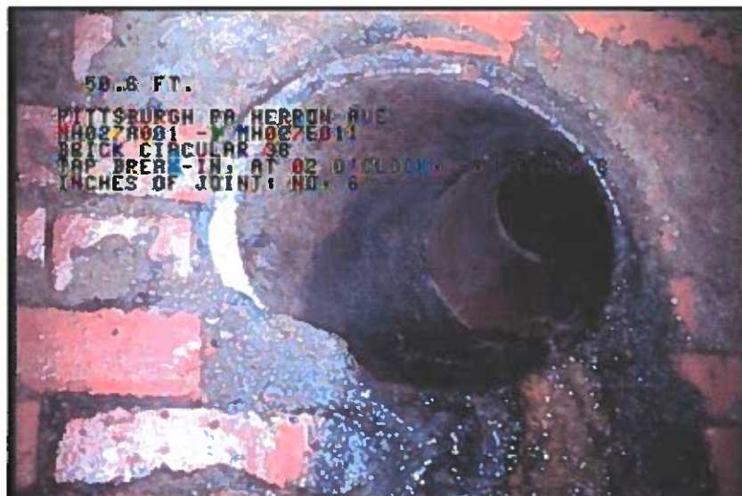
Photo: 1_7A, 00:08:18 50.6FT, Tap Break-In, at 02 o'clock, -, within 8 inches of joint: NO, 6"
