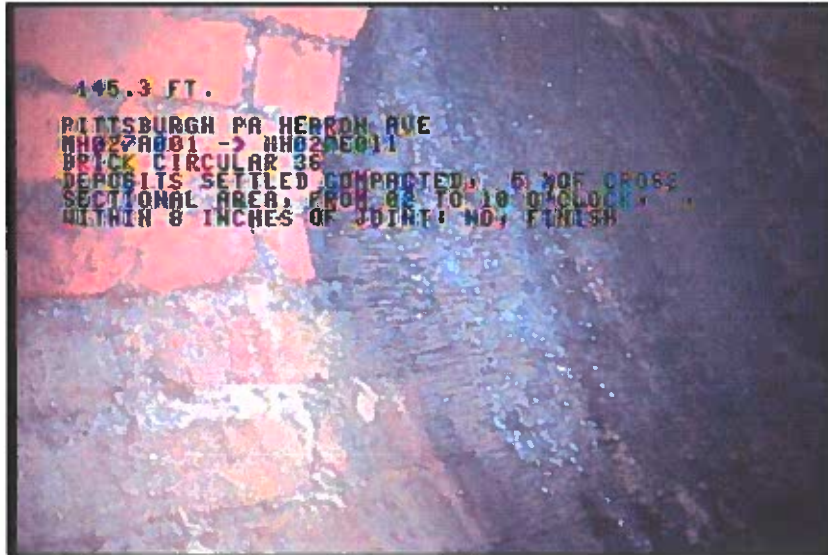
Photo: 1_12A, 00:13:24 145.3FT, Deposits Settled Compacted, 5 %of cross sectional area, from 02 to 10 o'clock, , within 8 inches of joint: NO, Finish
