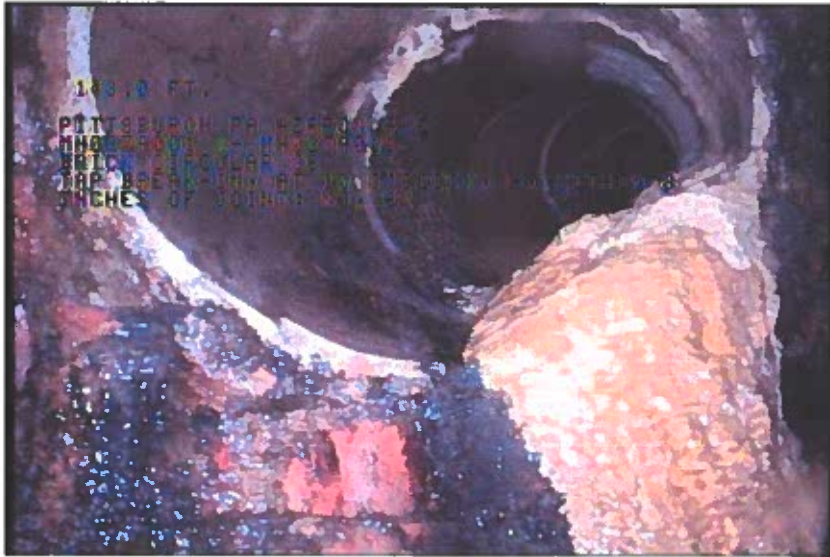
Photo: 3_8A, 00:07:41 143FT, Tap Break-In, at 10 o'clock, -, within 8 inches of joint: NO, 6" / DEPOSITES
