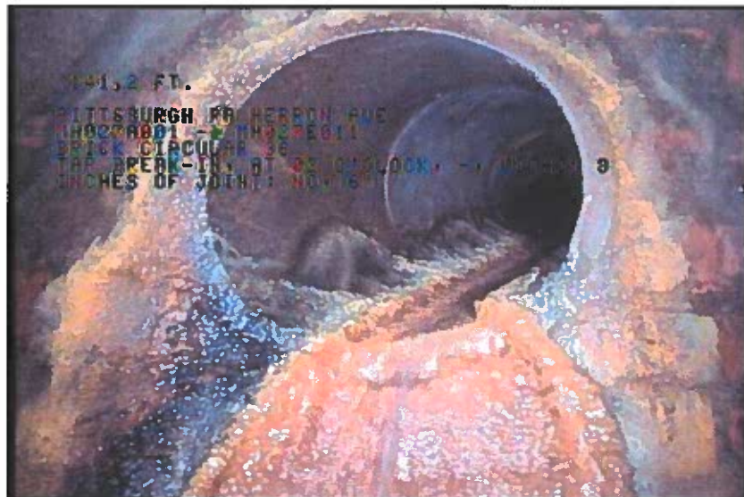
Photo: 1_11A, 00:11:46 141.2FT, Tap Break-In, at 02 o'clock, -, within 8 inches of joint: NO, 6"
