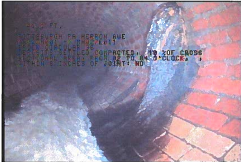
Photo: 1_6A, 00:07:39 41.1FT, Deposits Settled Compacted, 10 %of cross sectional area, from 02 to 04 o'clock, , within 8 inches of joint: NO / INFILTRATION
