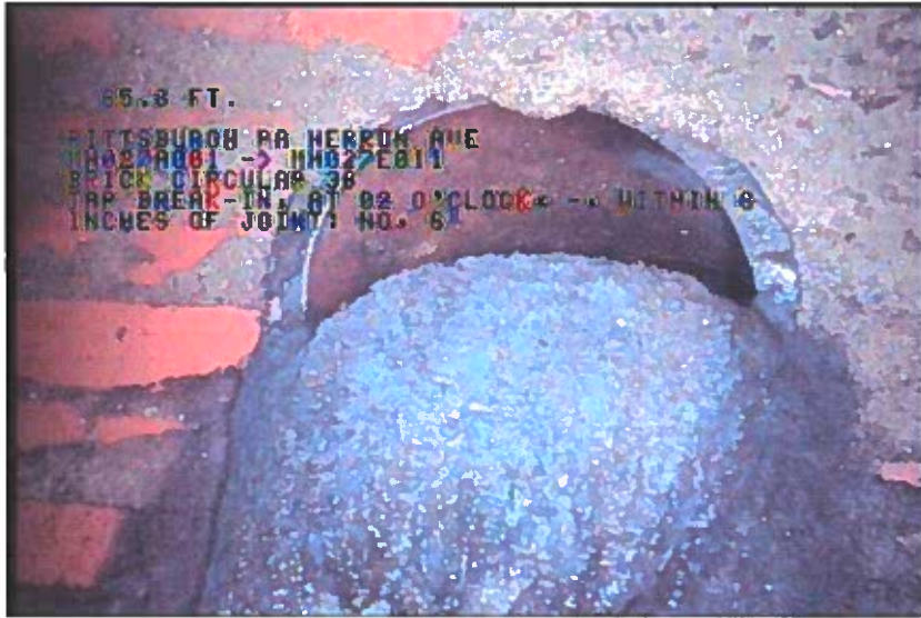
Photo: 1_8A, 00:09:05 65.8FT, Tap Break-In, at 02 o'clock, -, within 8 inches of joint: NO, 6" / DEPOSITES
