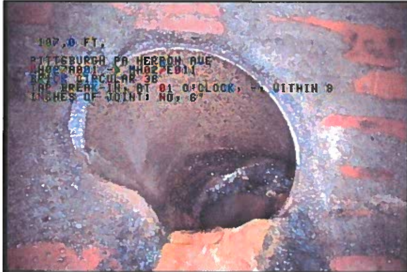
Photo: 1_10A, 00:10:49 107FT, Tap Break-In, at 01 o'clock, -, within 8 inches of joint: NO, 6"
