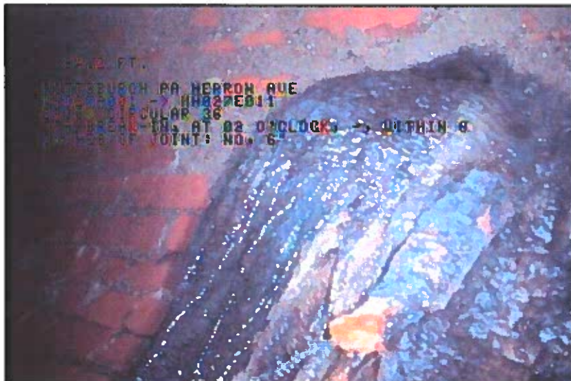
Photo: 1_9A, 00:10:05 84.2FT, Tap Break-In, at 02 o'clock, -, within 8 inches of joint: NO, 6" / DEPOSITES
