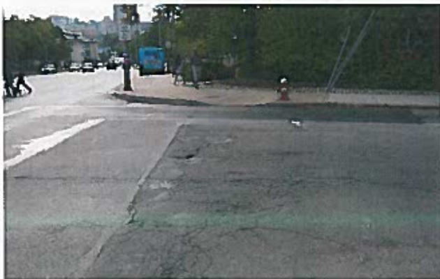
Lack of Pavement Markings
