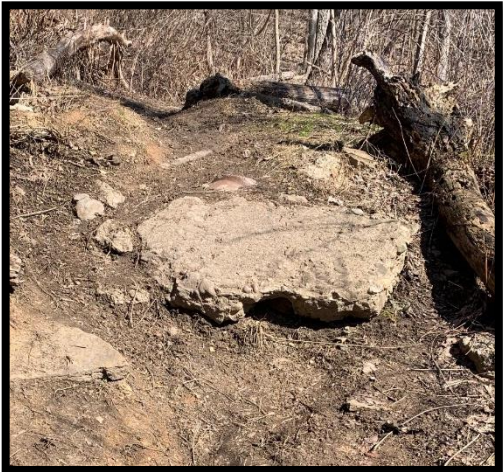
Figure 3: Concrete protruding from Concrete Block Trail
