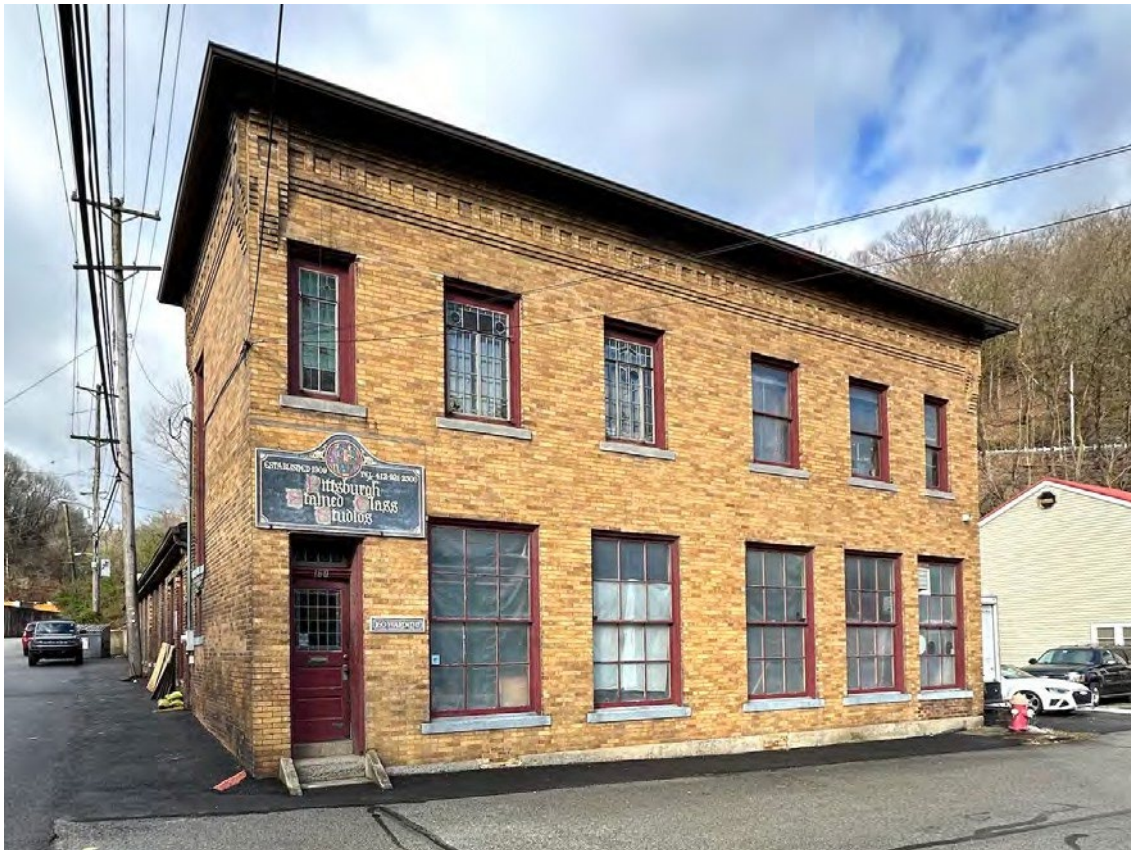
Photo 1. Front/east facade, looking northwest, showing the public entrance to the building on the left (Kirk Weaver, March 27, 2024).
