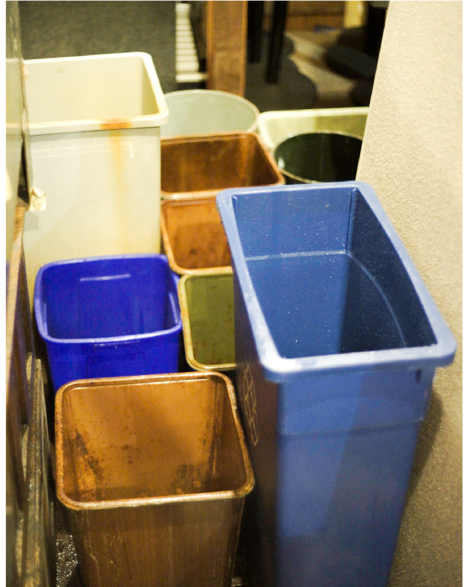
Buckets collecting water during a recent leak in basement storage.
