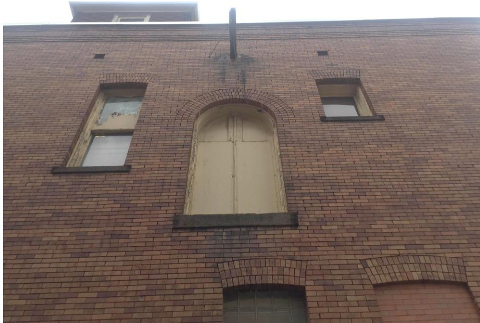
Photograph 3. Pittsburgh EMS Station, Culloden Way Facade, Southern Hayloft, Facing Northeast. Source: Calvin A Yoder.
