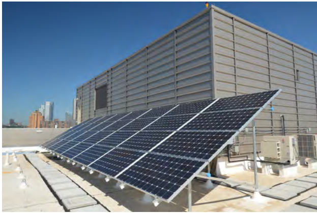
Photovoltaic panels on the roof of Des Places Residence Hall
