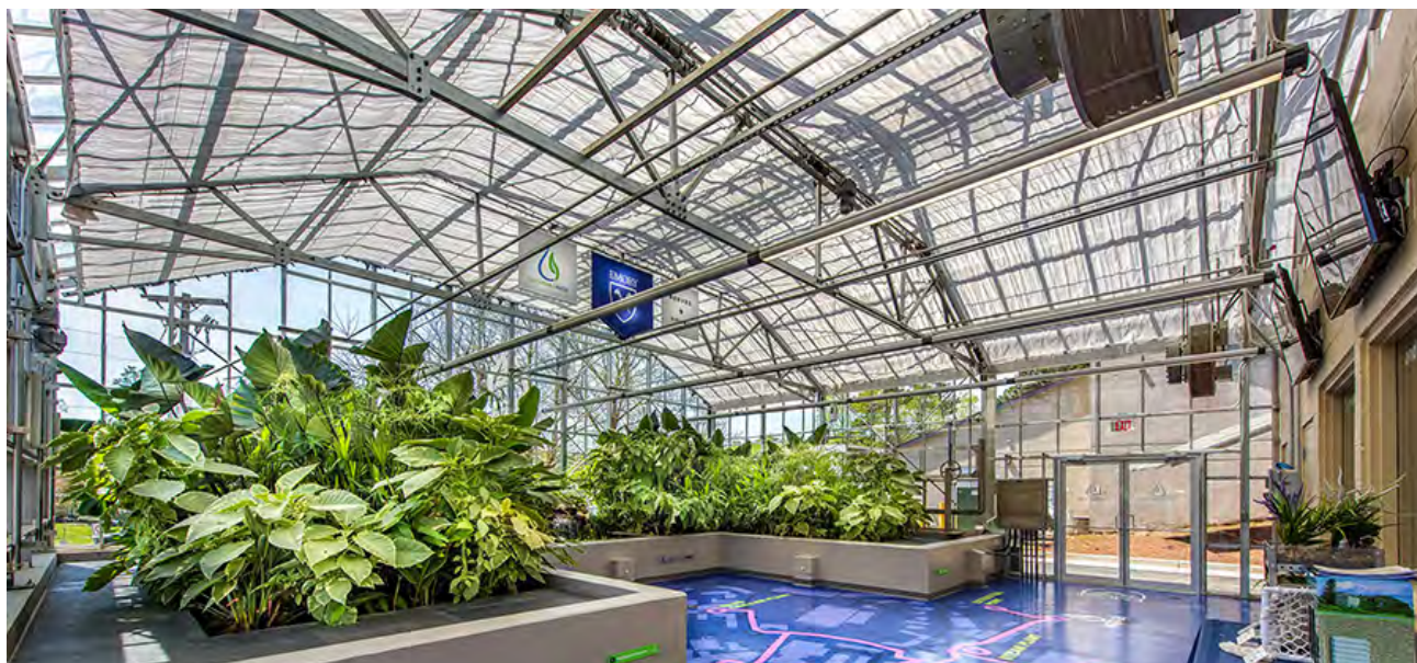
Interior photo of WaterHub® wastewater reclamation and reuse system at Emory University
