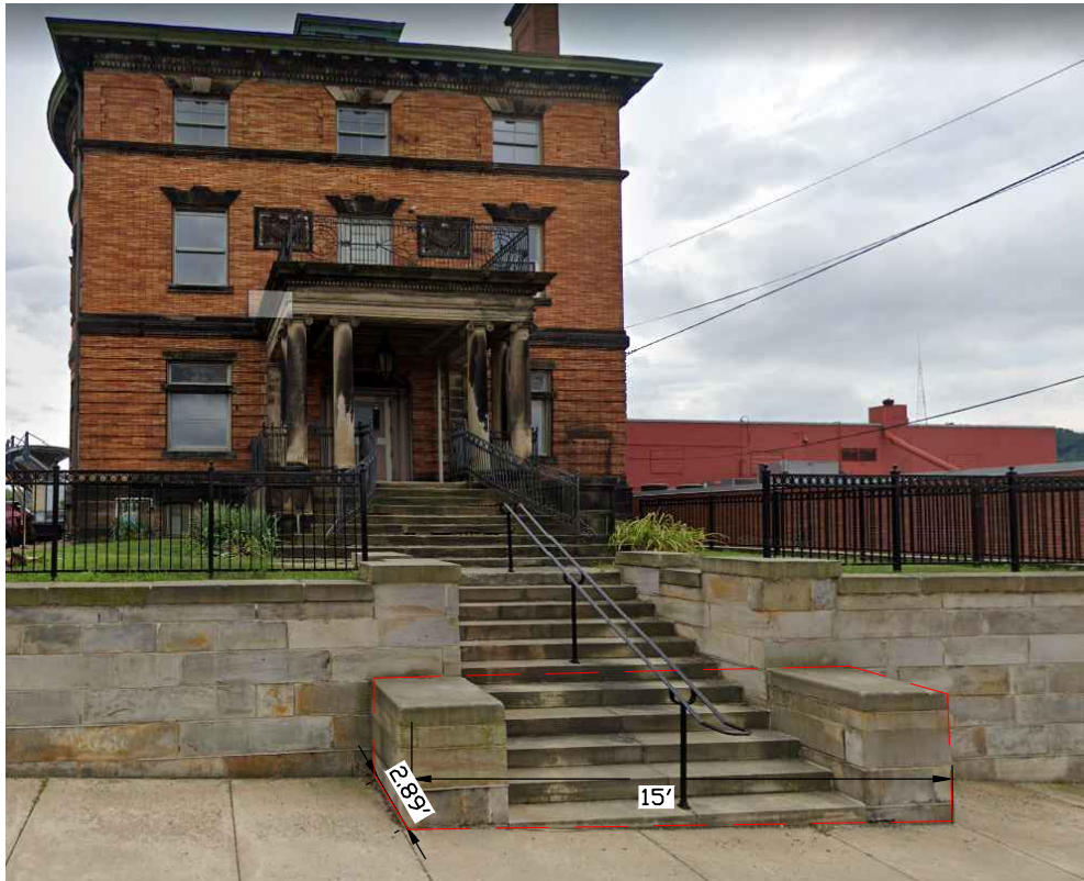
INSET IMAGE 1 : EXISTING STEPS ENCROACHING ON RIDGE AVENUE RIGHT-OF-WAY
