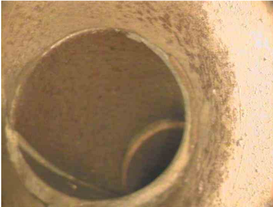
13, 00:04:23, 114.00ft Tap Factory Made at 1 o'clock, 6inch dim
