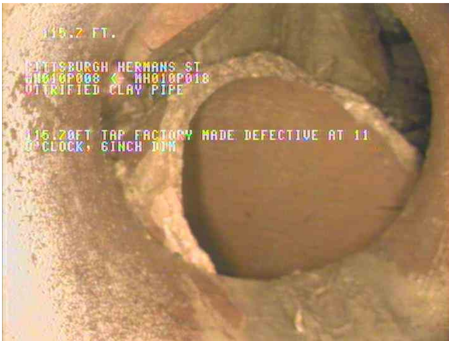
14, 00:04:36, 115.70ft Tap Factory Made Defective at 11 o'clock, 6inch dim
