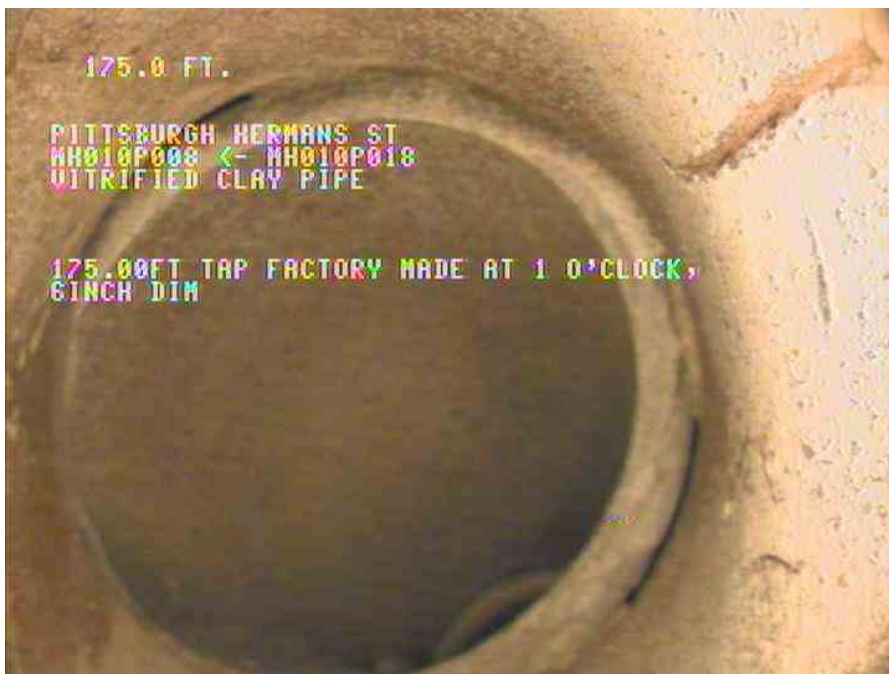
22, 00:06:53, 175.00ft Tap Factory Made at 1 o'clock, 6inch dim
