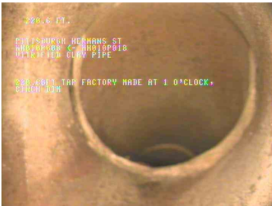
26, 00:09:35, 220.60ft Tap Factory Made at 1 o'clock, 6inch dim
