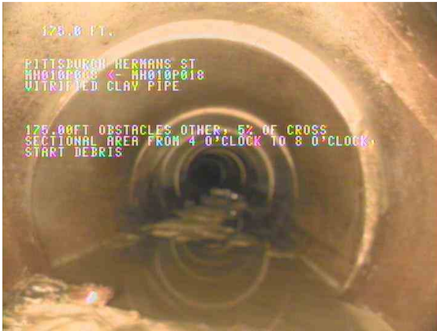
21, 00:06:45, 175.00ft Obstacles Other, 5% of cross sectional area from 4 o'clock to 8 o'clock, Start / DEBRIS
