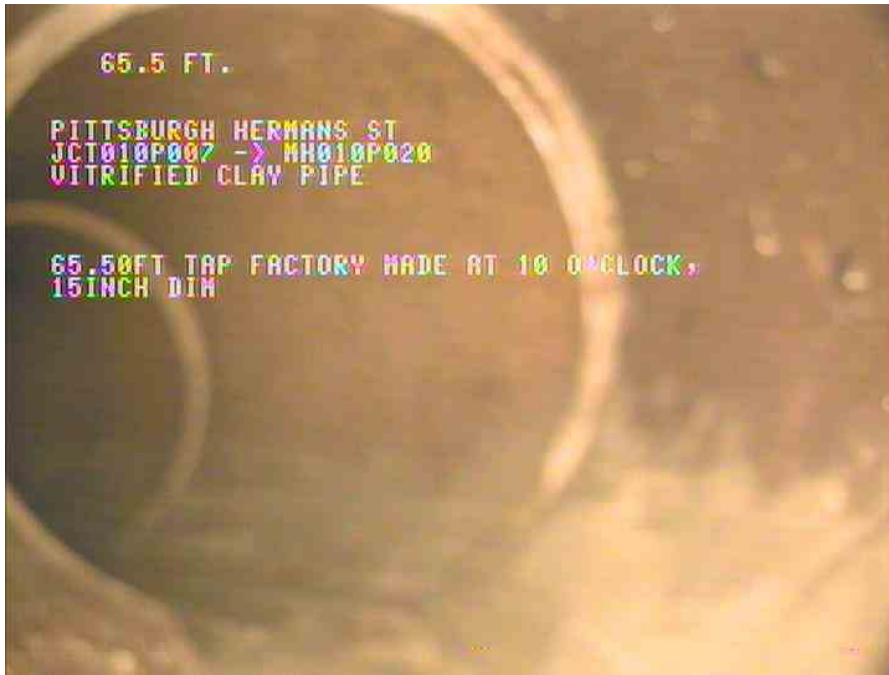
13, 00:04:10, 65.50ft Tap Factory Made at 10 o'clock, 15inch dim
