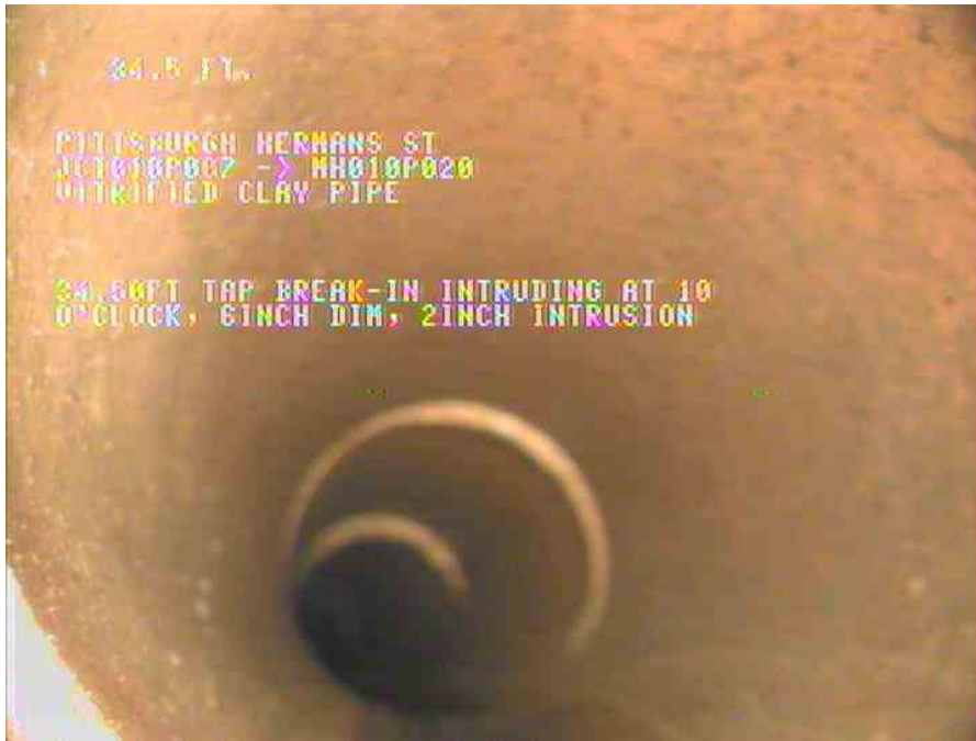
7, 00:02:24, 34.50ft Tap Break-In Intruding at 10 o'clock, 6inch dim, 2inch intrusion
