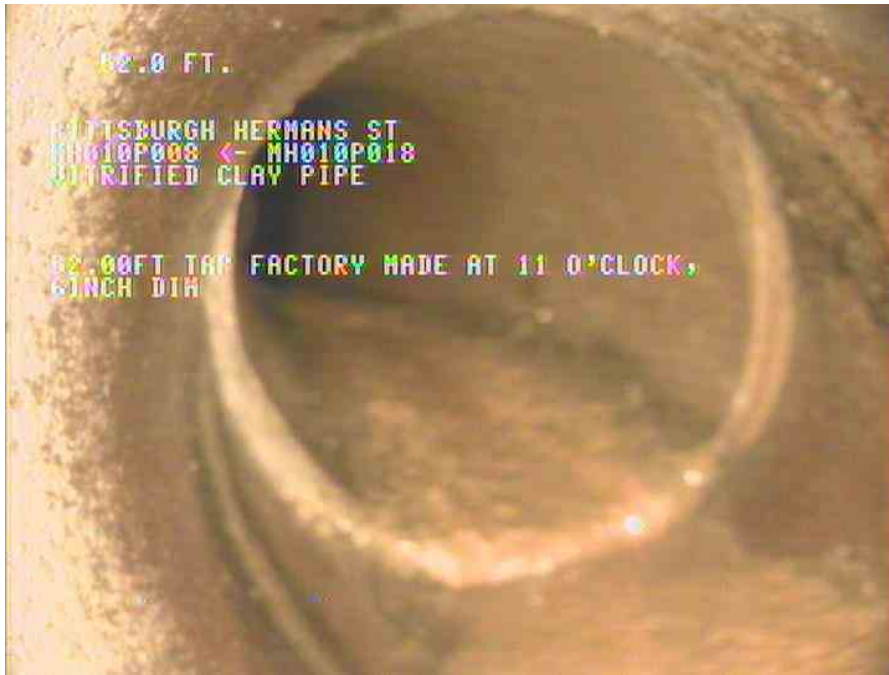
7, 00:02:32, 52.00ft Tap Factory Made at 11 o'clock, 6inch dim
