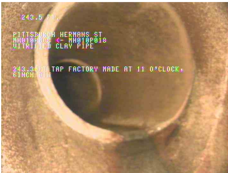
28, 00:10:14, 243.30ft Tap Factory Made at 11 o'clock, 6inch dim
