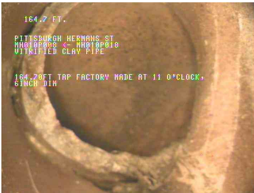
20, 00:06:16, 164.70ft Tap Factory Made at 11 o'clock, 6inch dim
