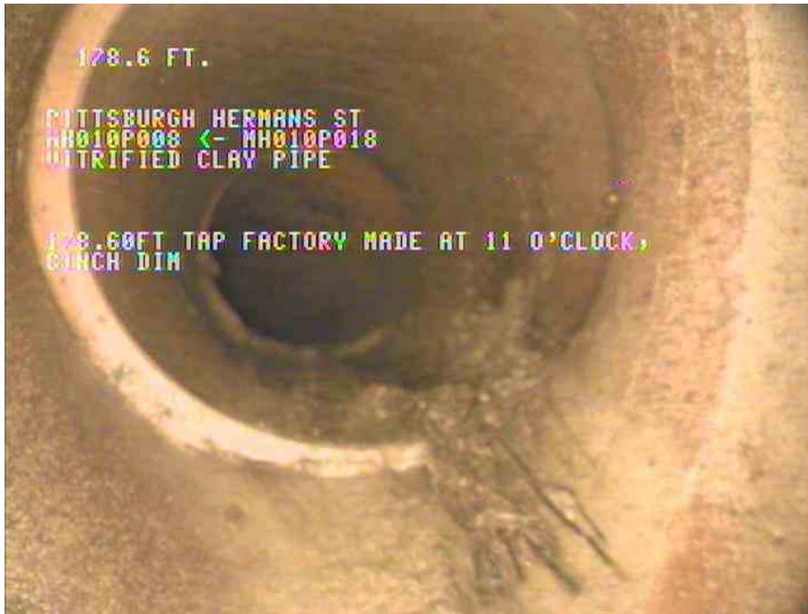
23, 00:07:08, 178.60ft Tap Factory Made at 11 o'clock, 6inch dim
