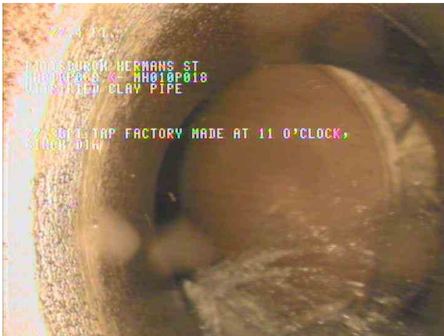
10, 00:03:25, 77.30ft Tap Factory Made at 11 o'clock, 6inch dim
