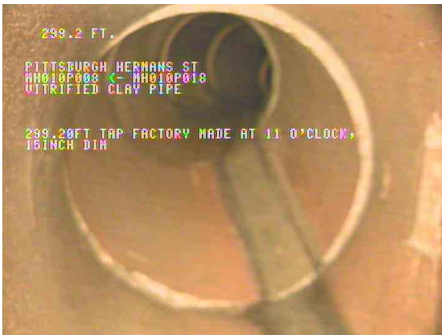
36, 00:12:32, 299.20ft Tap Factory Made at 11 o'clock, 15inch dim
