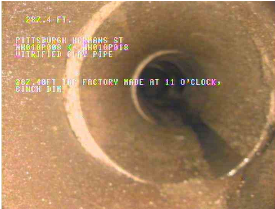
35, 00:12:00, 287.40ft Tap Factory Made at 11 o'clock, 6inch dim
