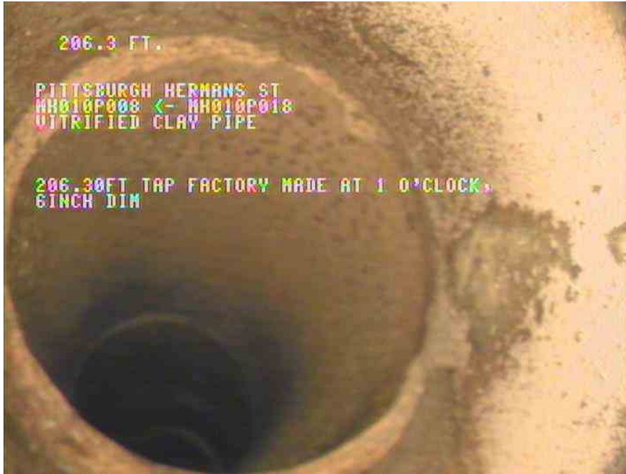
25, 00:09:06, 206.30ft Tap Factory Made at 1 o'clock, 6inch dim
