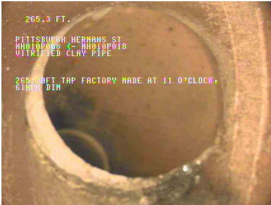
31, 00:11:07, 265.30ft Tap Factory Made at 11 o'clock, 6inch dim
