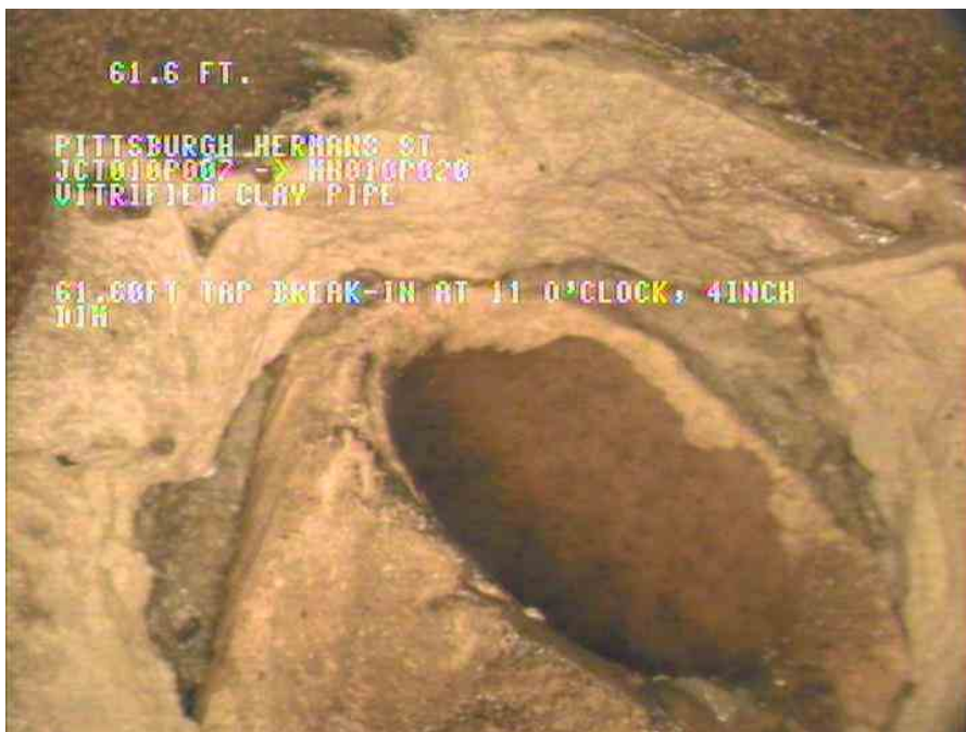
12, 00:03:48, 61.60ft Tap Break-In at 11 o'clock, 4inch dim
