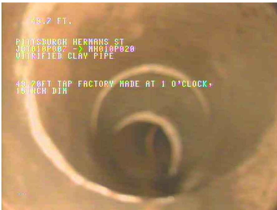
10, 00:03:04, 49.70ft Tap Factory Made at 1 o'clock, 15inch dim
