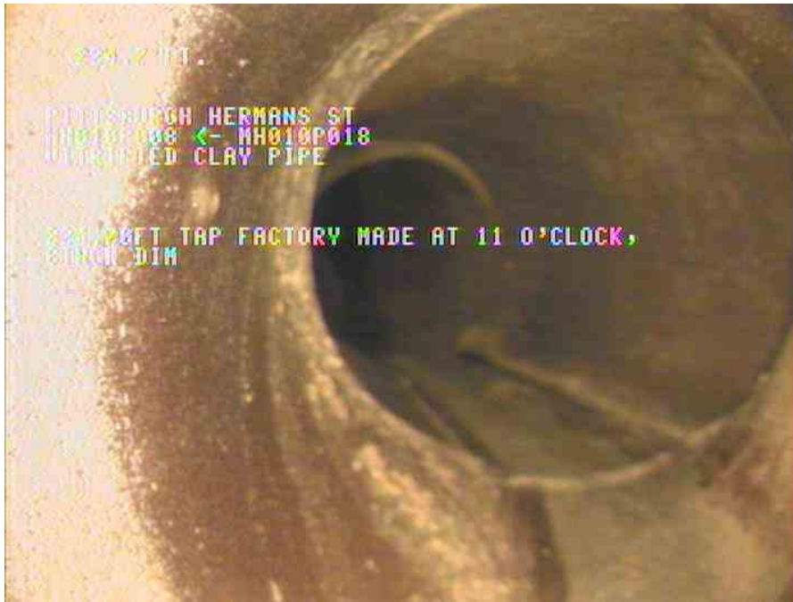
27, 00:09:47, 224.70ft Tap Factory Made at 11 o'clock, 6inch dim
