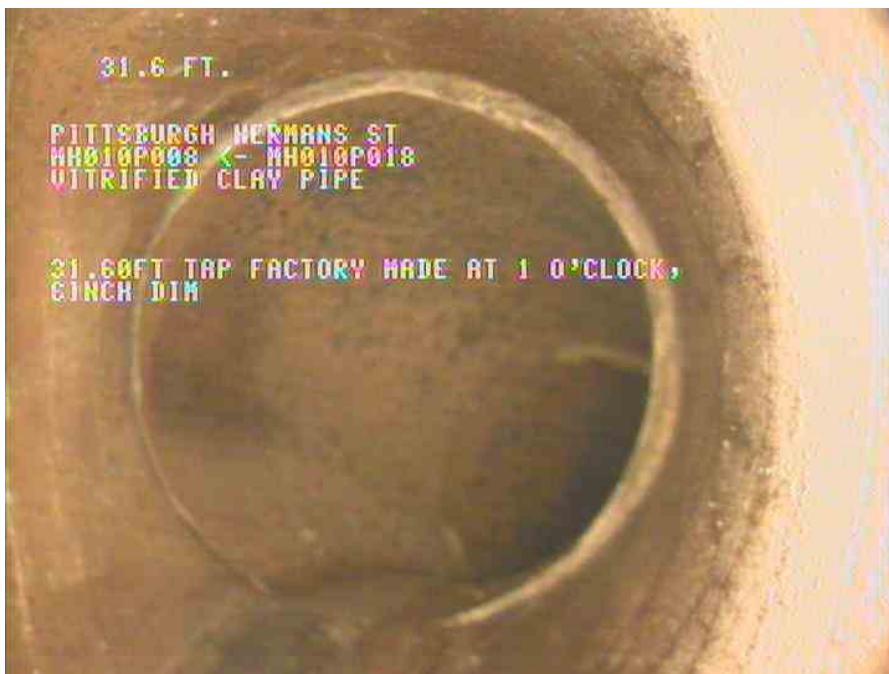
4, 00:01:46, 31.60ft Tap Factory Made at 1 o'clock, 6inch dim
