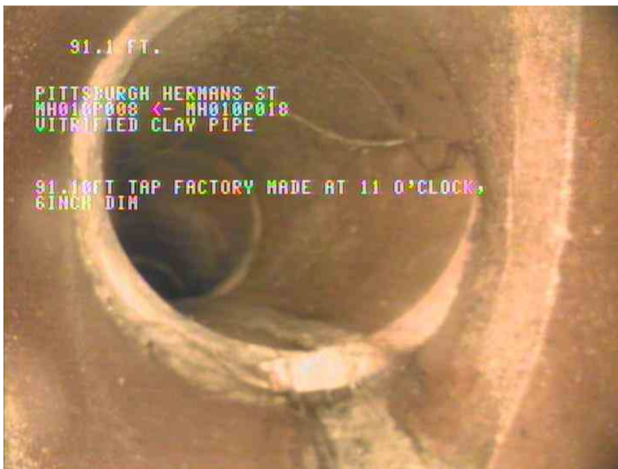
12, 00:03:53, 91.10ft Tap Factory Made at 11 o'clock, 6inch dim
