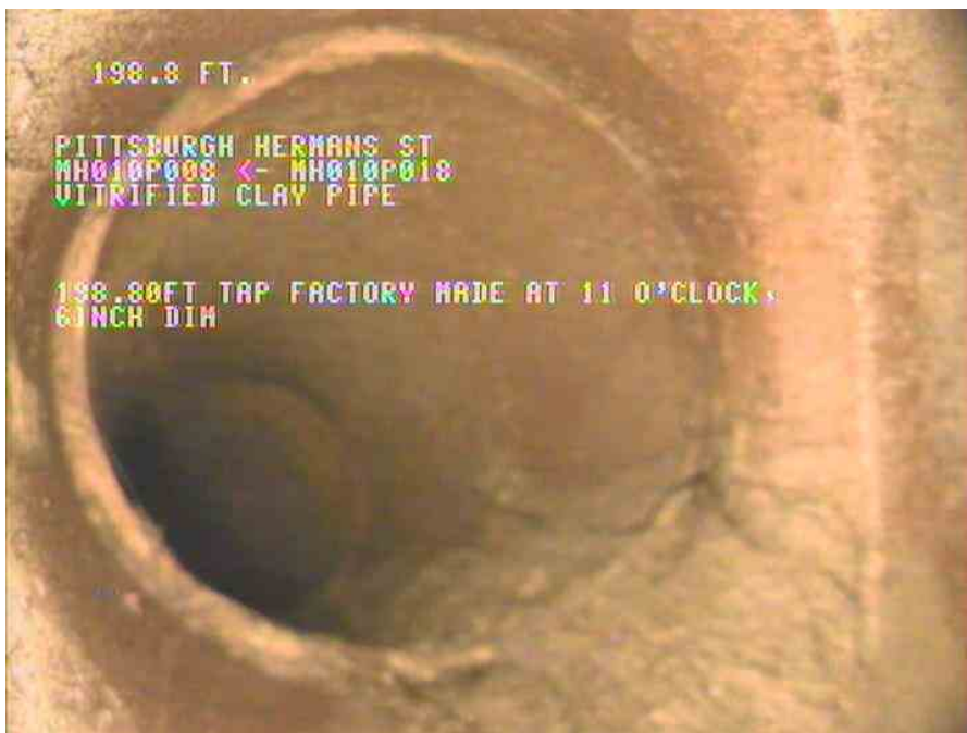
24, 00:08:47, 198.80ft Tap Factory Made at 11 o'clock, 6inch dim
