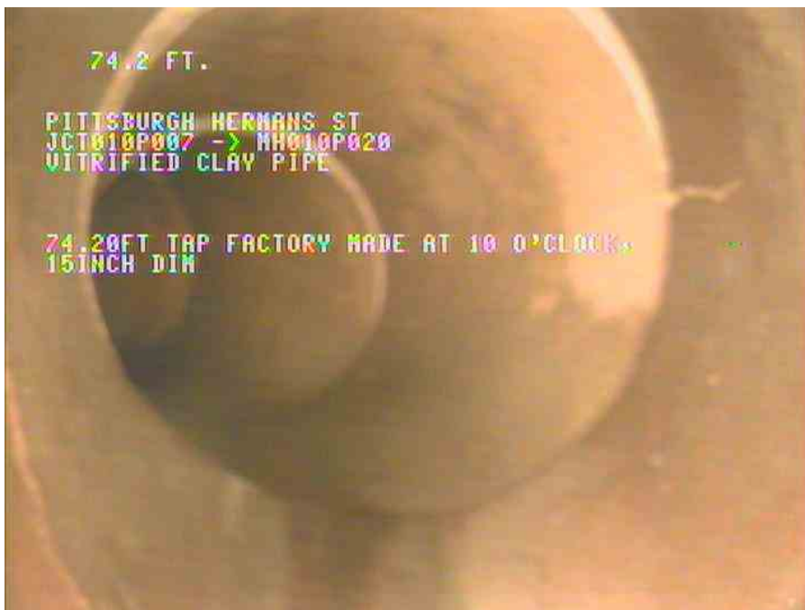
14, 00:04:37, 74.20ft Tap Factory Made at 10 o'clock, 15inch dim
