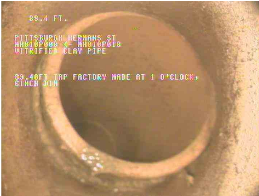
11, 00:03:44, 89.40ft Tap Factory Made at 1 o'clock, 6inch dim
