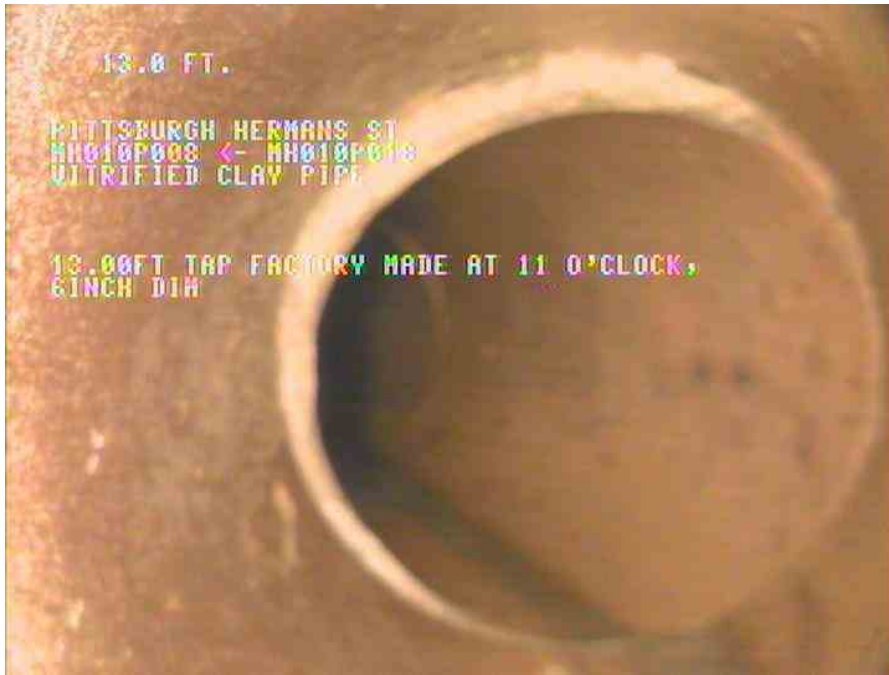
3, 00:01:21, 13.00ft Tap Factory Made at 11 o'clock, 6inch dim
