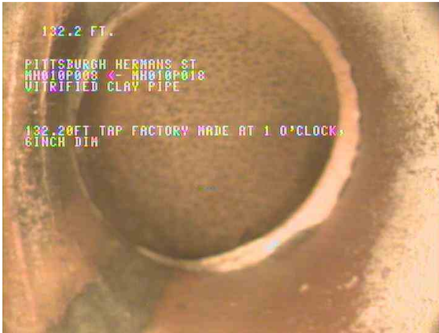
15, 00:04:59, 132.20ft Tap Factory Made at 1 o'clock, 6inch dim
