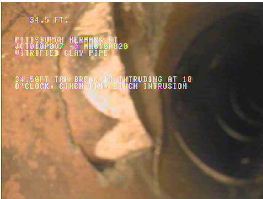
8, 00:02:24, 34.50ft Tap Break-In Intruding at 10 o'clock, 6inch dim, 2inch intrusion
