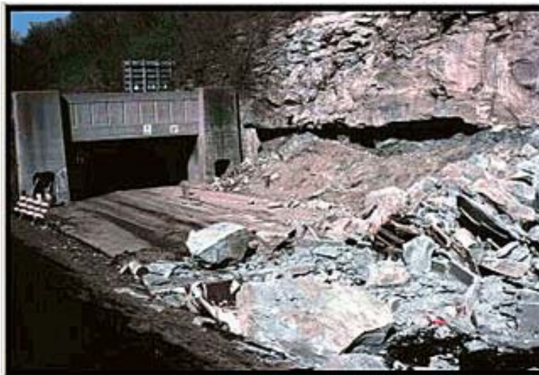
Figure 3.3: Rockslide at Wabash Tunnel
