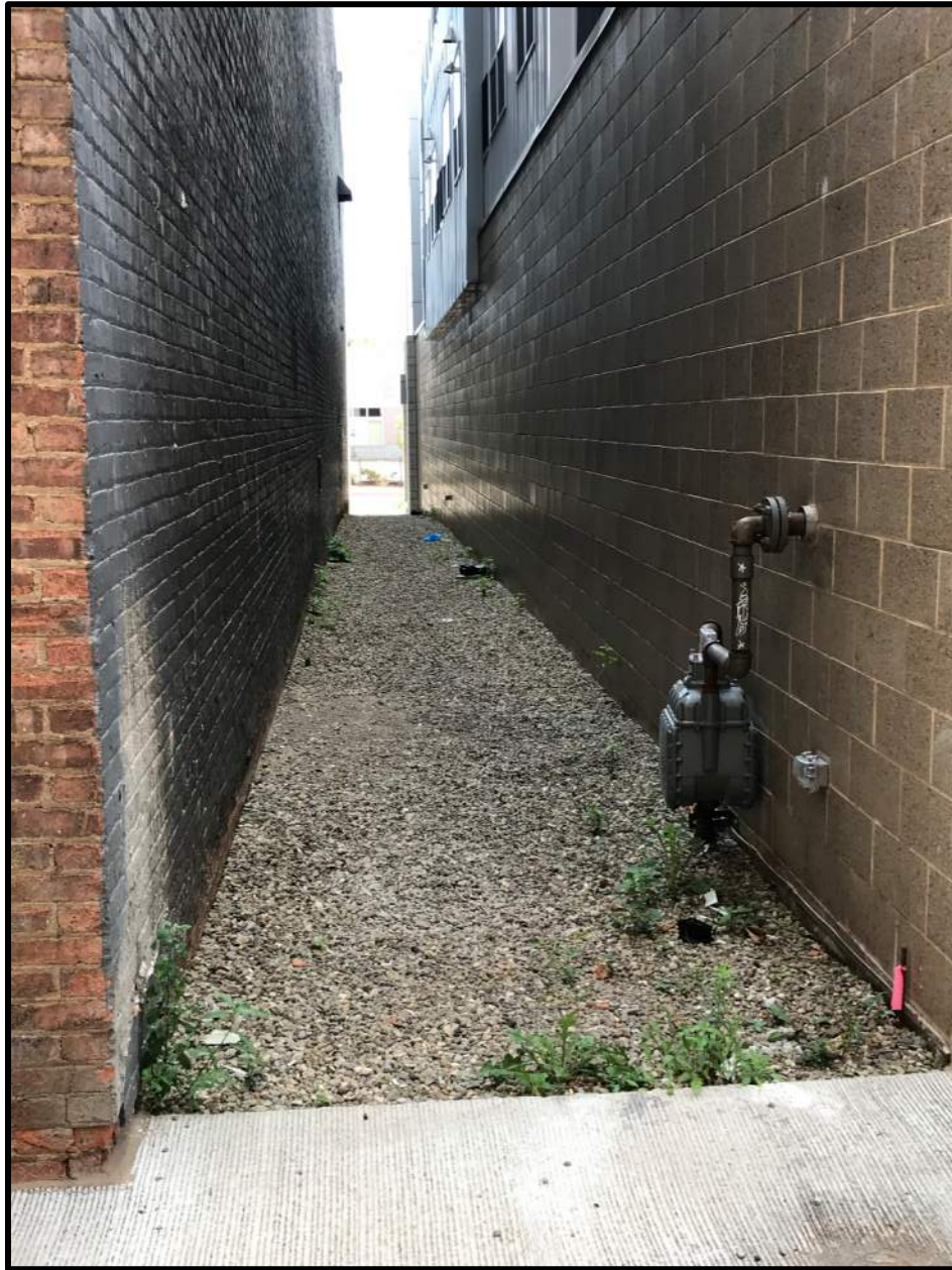
Figure 7. Side of building on Commerce Street looking south-east adjacent to Emerald Apartments
